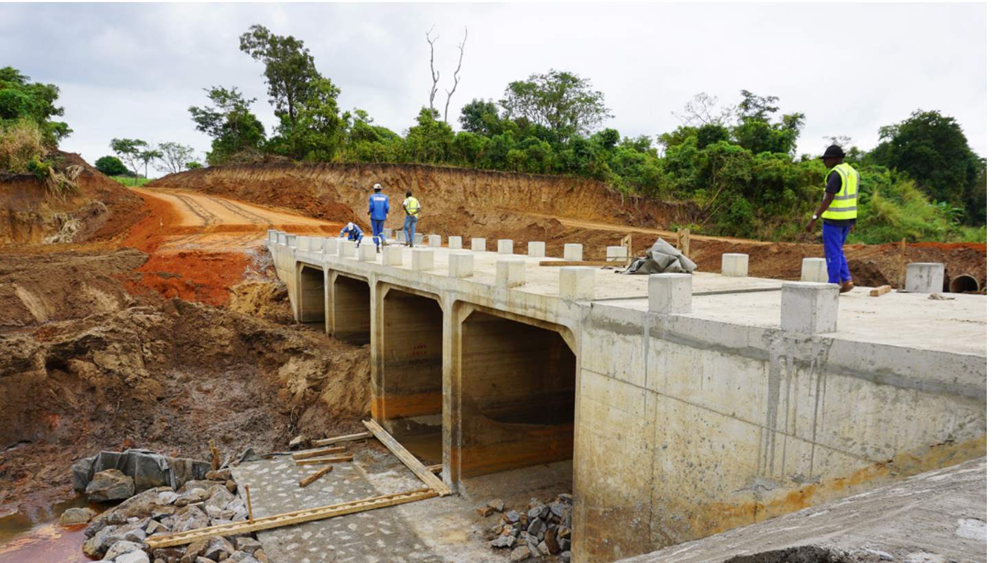
Two bridges were constructed and the road was improved in order to make the replacement land more accessible to the PAPs. Photo: Norfund
